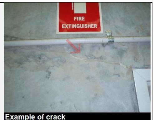
Example of crack
